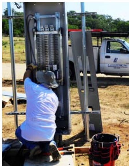
L&O Electric has donated and completed all of the electrical infrastructure for the entire main campus
