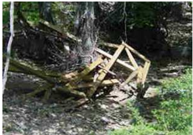
Tangled bridge wreckage after the floods came down the creek
